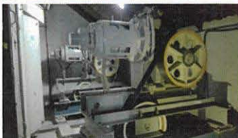
Lift 1 & 2 - Roof Motor Room
