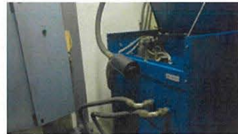
Lift 3 – B3 Hydraulic Machine Room
